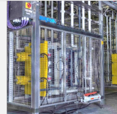
Design and realization of a low cost Electrodialysis module for brackish water desalination plants
